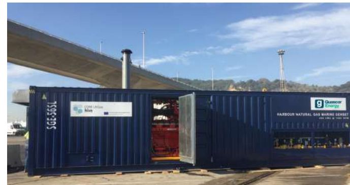
Containerized 56SL genset for harbour use.
