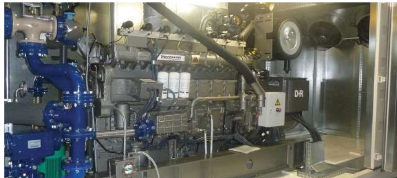
A CHP package of SM genset.
