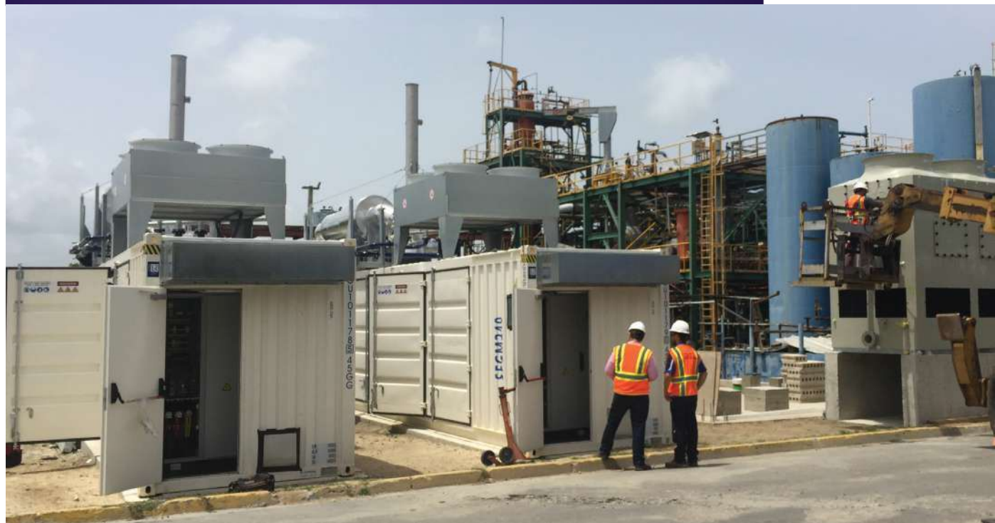
Olein food industry plant, two containerized G-24SM engines.
