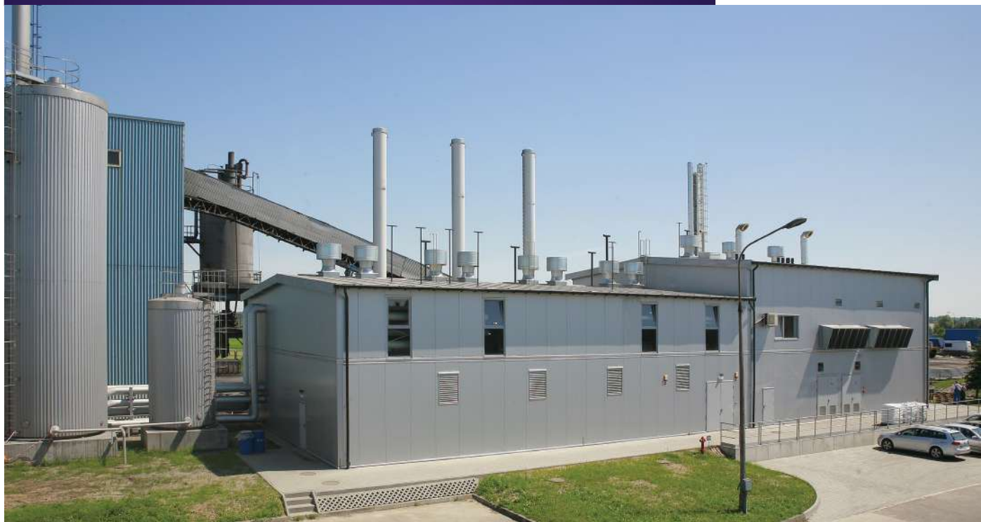
Condensation plant - Sokołowie Podlaskim - Poland.
